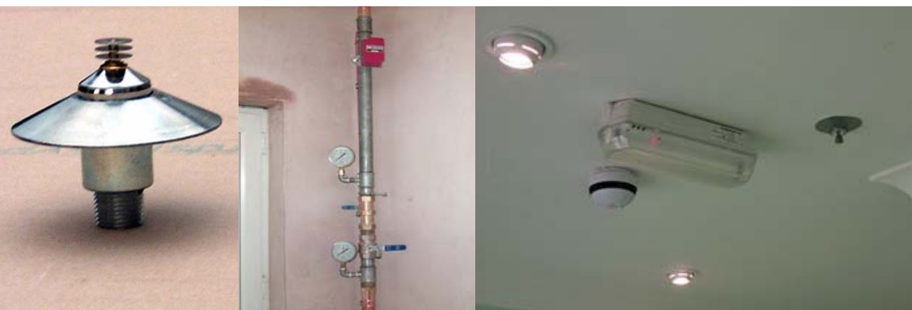
The system was fitted with Institutional heads similar to the one shown above
