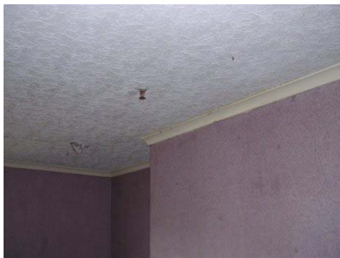
Fig 6 One of the sprinkler heads this one is in front of the chimneybreast
