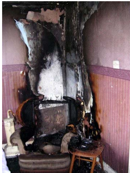
Fig 7 Test 2 after fire, chimneybreast s to the left
